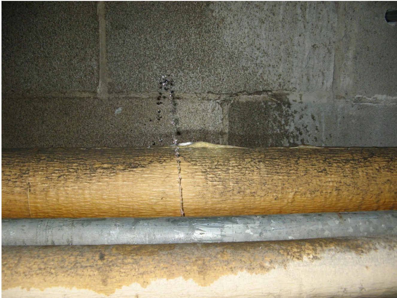
Leaking Galvanized Piping
